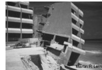
Eroded foundation and resulting collapse of a building on the coast following a hurricane-induced storm surge
