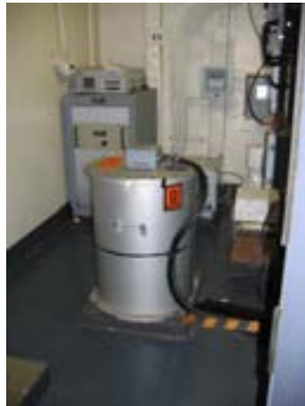
Photo 12: The Gyro Compass is stored below on the Deck 3.
